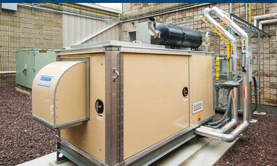
The new generator sits outside the facility, while a new pump and heat exchanger were installed in the existing mechanical room.
